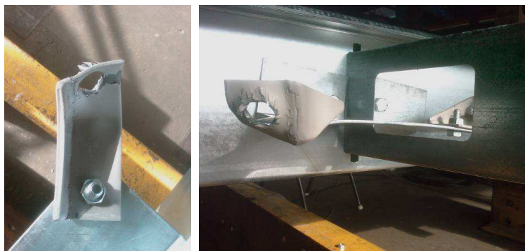
Figure 80. Failure mode t4)
