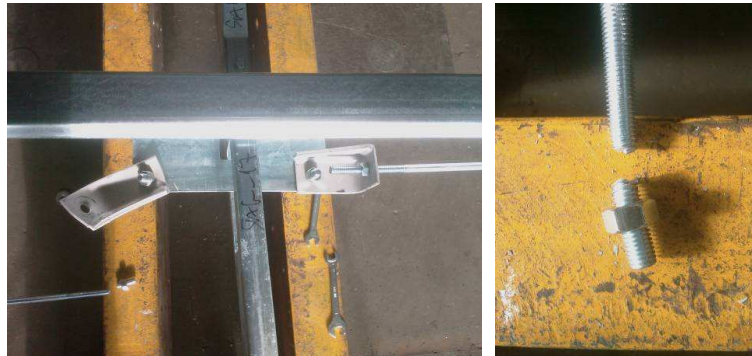
Figure 81. Failure mode t5)
