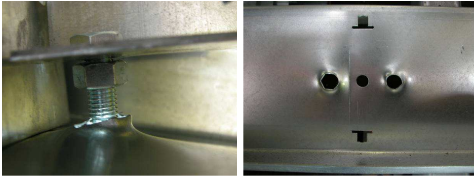
Figure 78. Failure mode t2)
