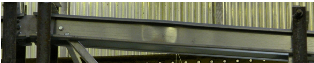
Figure 80.: Buckling of the web in the upper chord.
