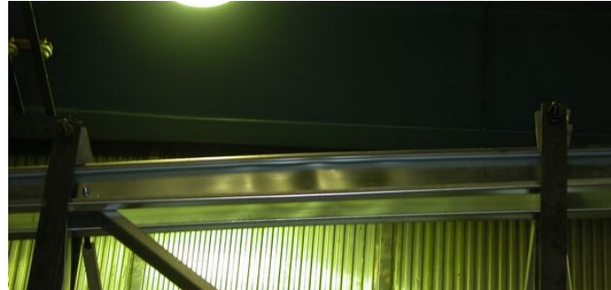
Figure 96.: Local buckling in the upper chord.
