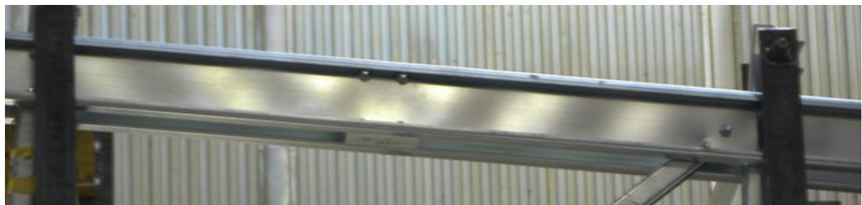
Figure 88.: Local buckling in the upper chord.
