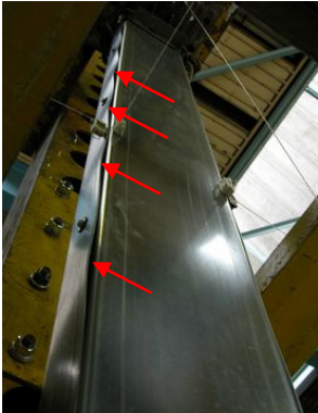
Figure 31.: Local buckling (CU).
