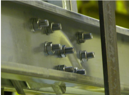
Figure 95.: Failure in the lower chord
