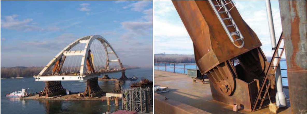
Figure 4.34: Erection of the arch bridge: (a) floating operation and (b) supporting bar details.
